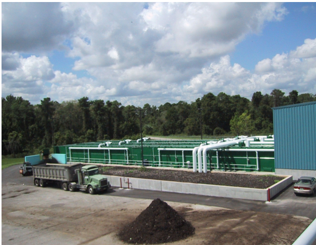
The Wright Environmental In-Vessel System.
